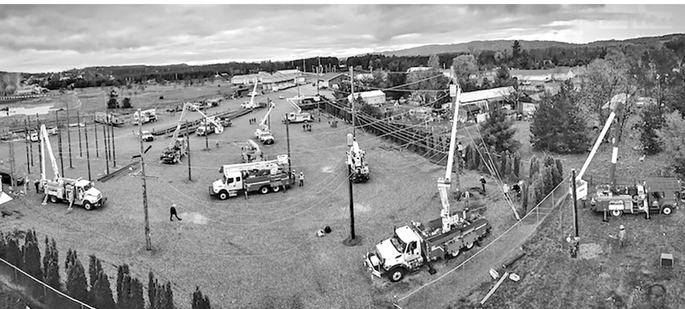
Lineworkers from Great Lakes Energy, Consumers Energy, Traverse City Light & Power, City of Charlevoix and Wolverine Power Cooperative volunteered their time Saturday to complete the J.H. Farrington Training Area, named in memory of Consumers lineworker James (Jim) Farrington who recently lost his life on the job. COURTESY PHOTO
